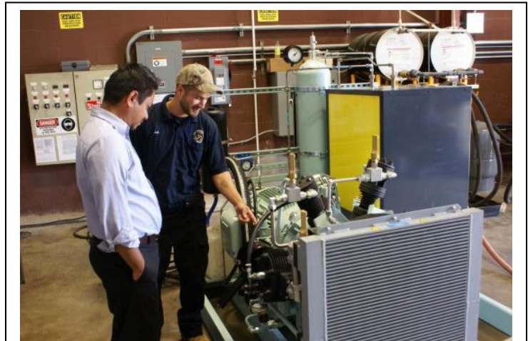
A strong maintenance program ensures long life and optimal performance of a plant's air compressors.
